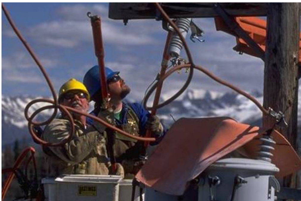
Image courtesy of Anchorage Municipal Light & Power.
